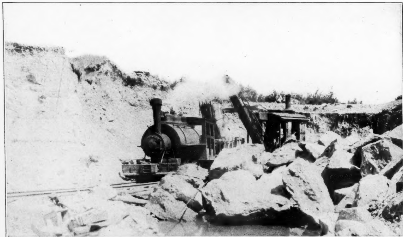
Upper Left—Close view of new crusher and train of cars from pit approaching the dumping place. Upper right—Elevator to sand bin and car about to be loaded from it. Lower—Locomotive and shovel at operation in the pit. Note large stones which the new crusher has been installed to break up.
